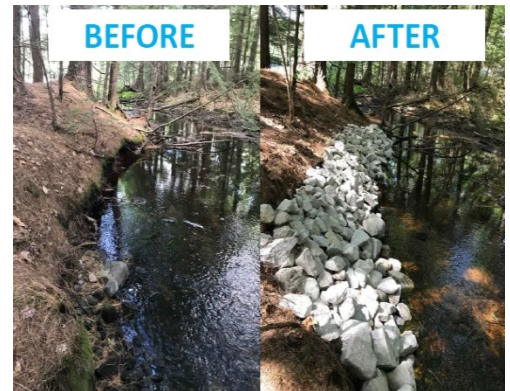
Riprap installed by 30MRWA's YCC stabilizes the soil and prevents it from washing into the stream.
